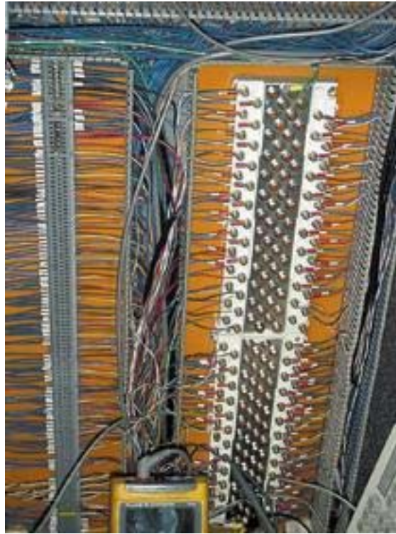
Figure #6: Carbon Block Suppressors
