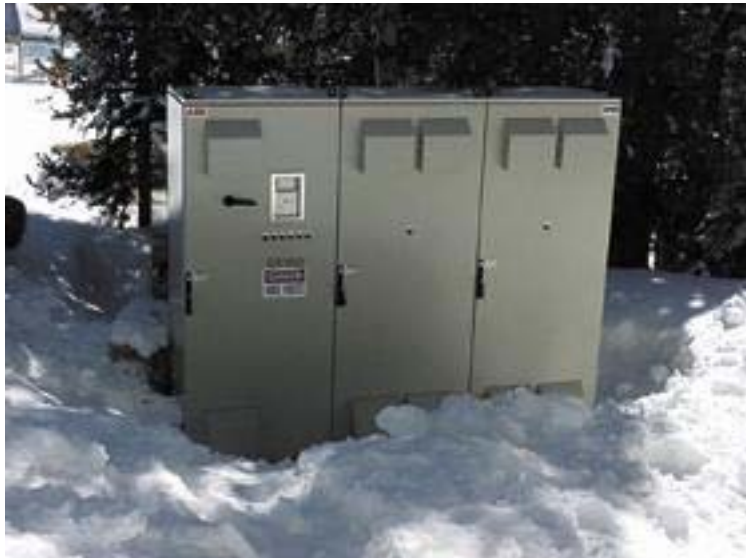
Figure #7: Chile Express Distribution System on Mountain Summit.
